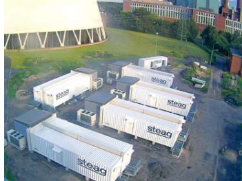
BESS (Battery Energy Storage System) system in Germany
