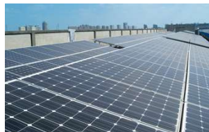
Solar panels installed on the roof of Nidec (Zhejiang) Corporation's building
