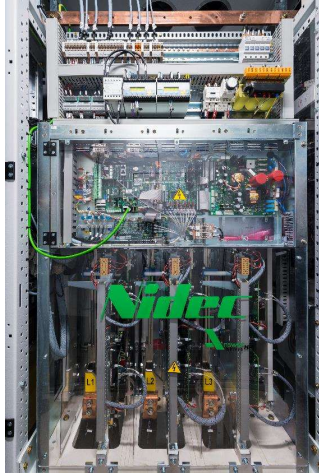
Power conversion system essential for BESS
