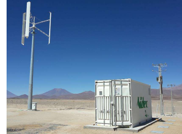
Micro-grid system in Chile
