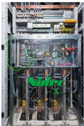
Power conversion system essential for BESS
