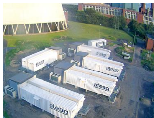
BESS (Battery Energy Storage System) system in Germany
