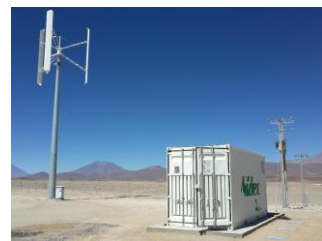
Micro-grid system in Chile
