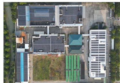
Solar power generation system installed at NIDEC PRECISION (ZHEJIANG)
