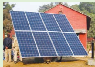
Nidec's first solar pump system installed in an Indian state-owned farm
