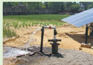
Nidec's second solar pump system installed in an Indian state-owned farm
