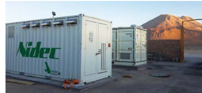
Micro-grid system in Chile
